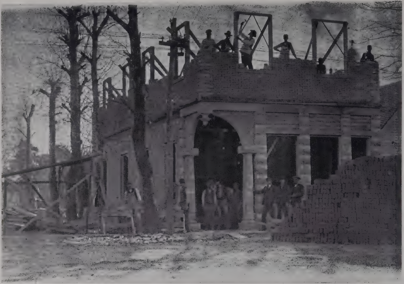
Building the Bank—Standing on the second floor at corner with trowel in hand, Emory M. Jennings; standing in window with hammer, Jim Collins, next with hand on wall, Charley Manwarring. On ground in doorway, Jim Cochran; with hand on pillar, Elza Jennings, and next to him, Rufus Jennings.
