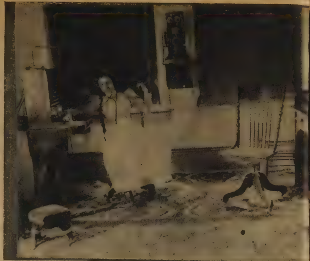
FIRST SWITCHBOARD in Opelousas, in the office of the Bertha Telephone Co., installed by Miss Isola Campbell, first operator. She was the late Mrs. A. S. J. Campbell. Bertha Telephone Co. was owned and installed by Allie Burton Pickett, of Wisconsin, married Vidalia Comeau and settled here. This photo of the early switchboard is a less collector's item. It offers an interesting contrast to the modern one in present photo. Note the old crank 'phone on the wall.
