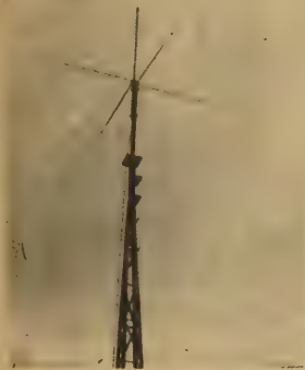
RADIO TOWER — enables us to keep in contact with our trucks at all times.
