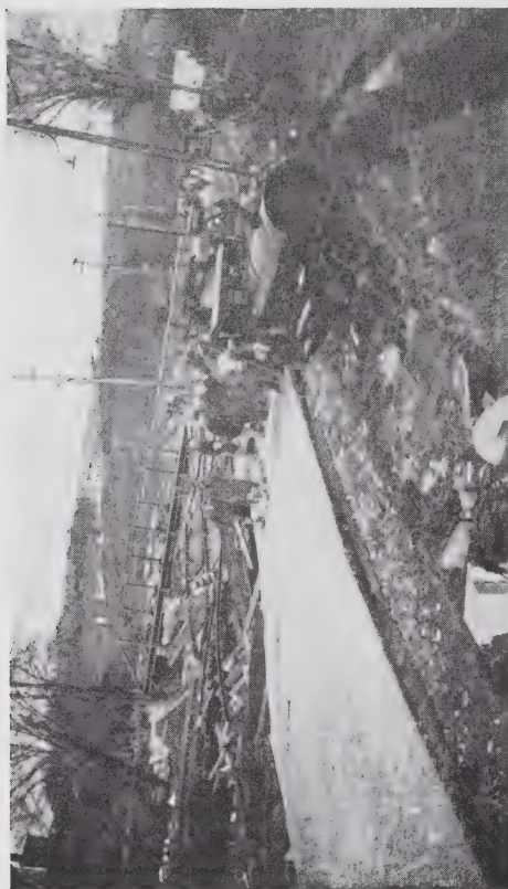
Heavy Trucks Hoisted Off the North Main Street Pavement and Deposited Beside the Road. Cement Pavement Was Broken At This Point.
